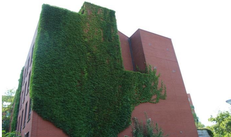
Image 7: Coarse vegetation on a building façade at GWL Terrain. Next boxes are also visible on the right side of this building (Author, June 3, 2018).
